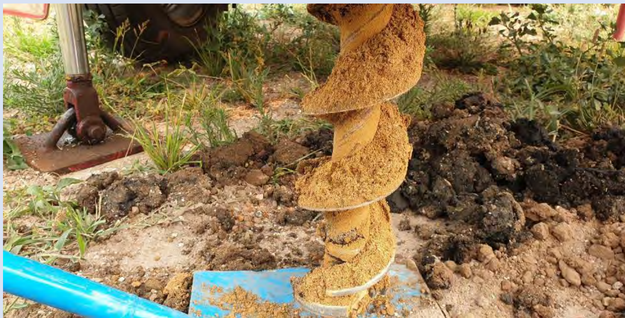
Photograph 14: Concrete and rubble in Fill
