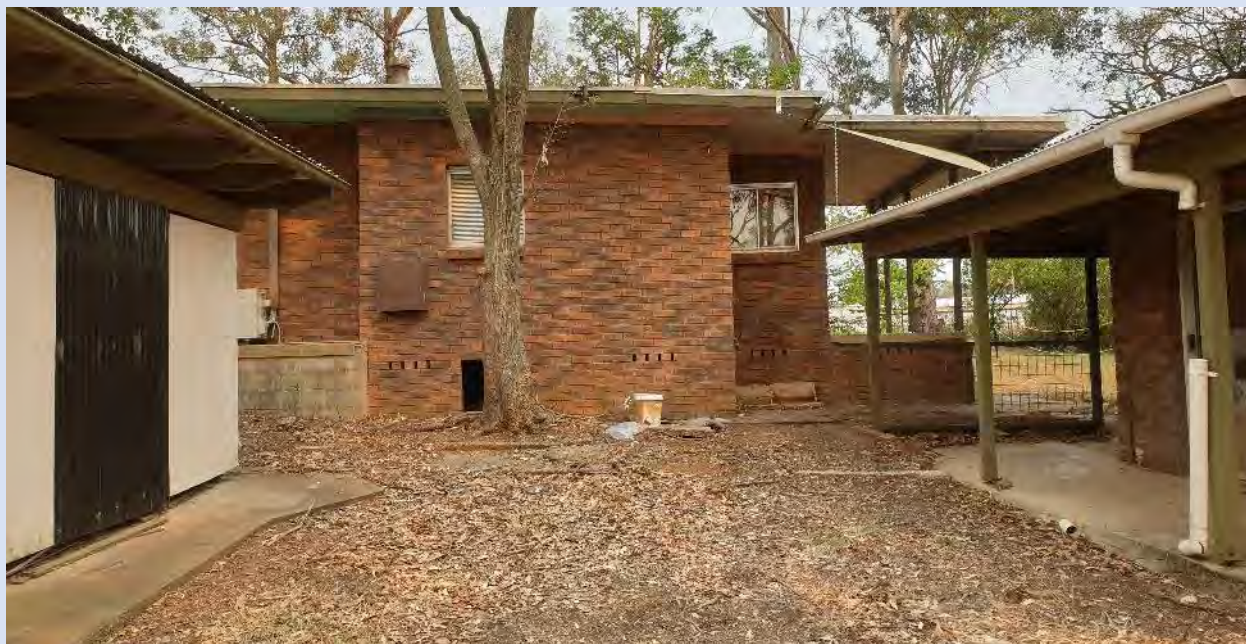
Photograph 11: Suspected Asbestos Fragments
